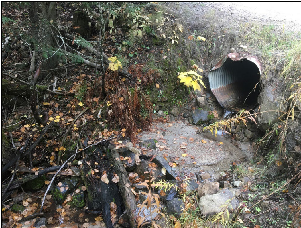
PHOTO 13. SAND FROM ROAD SURFACE ENTERS DUMONT CREEK AT SITE DT13.
